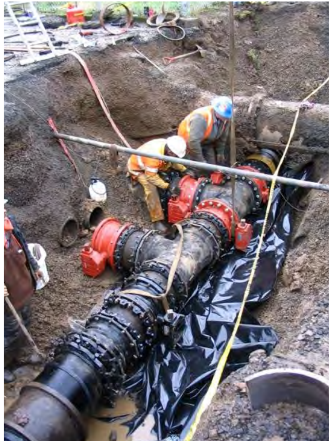
Newberg's Public Works Department has plenty of infrastructure work for its crews
