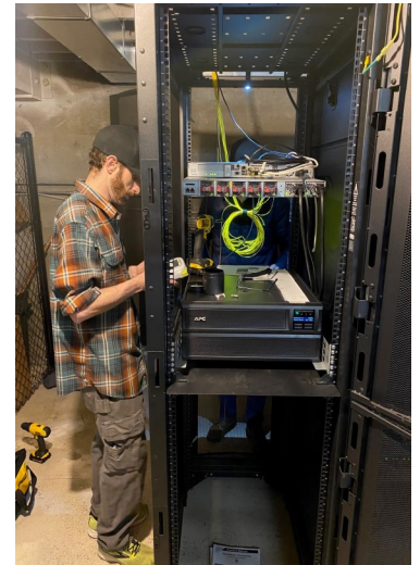
City of Pendleton IT Technician working on relocating City's internet firewall to a new Internet Service Provider (ISP) location.
