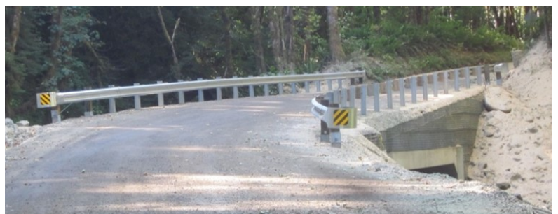
Figure 9. Streambed restored and road fill being constructed. The pedestal footing is still exposed at final streambed elevation.
