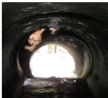
Figure 1. Separated culvert joint.
