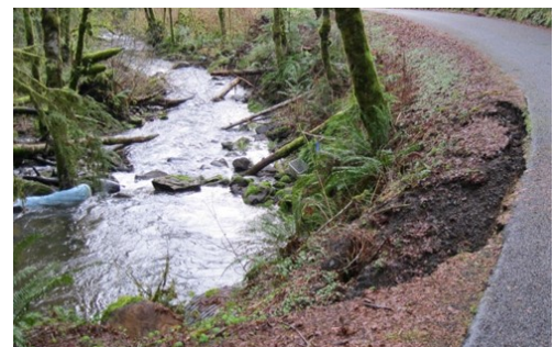
Figure 2. Road fill failure and mattress in the background.
