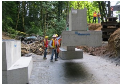
Figure 8. Setting precast elements on the GRS foundation. Note the apparent load capacity of the mat compared to Figure 5.
