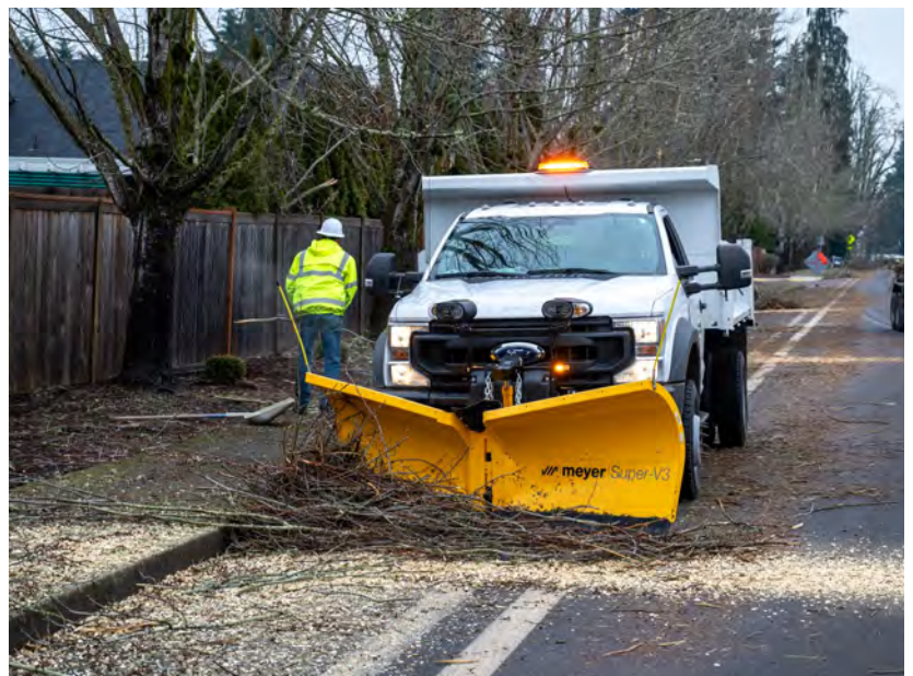
Snow plows quickly become "tree debris plows" for Springfield Operations crews dealing with thousands of trees damaged from heavy ice.
