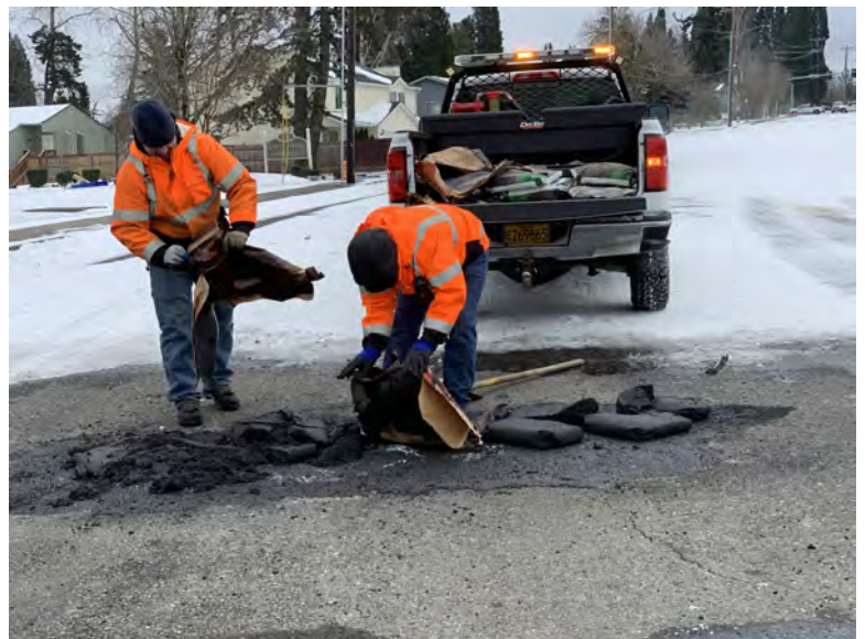
A downed utility line liquified and melted a section of pavement on one of Gresham's busier arterials. After the line was made safe and removed, City of Gresham Transportation Operations crews patched the pavement to re-open the road to traffic.
