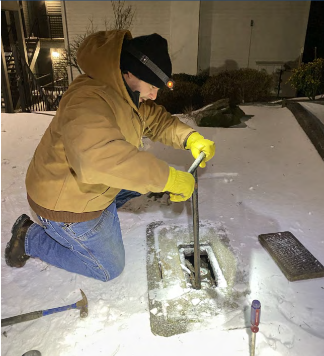
In Lake Oswego, two water crew heroes put their bodies on the line hand digging a 4 ft. deep trench with a pick ax to repair a broken water main in 15F temperatures.
