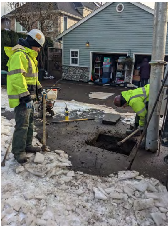
Public Works crew members assisted more than 300 water shut-offs in extreme conditions due to freezing or burst pipes in the City of Lake Oswego.
