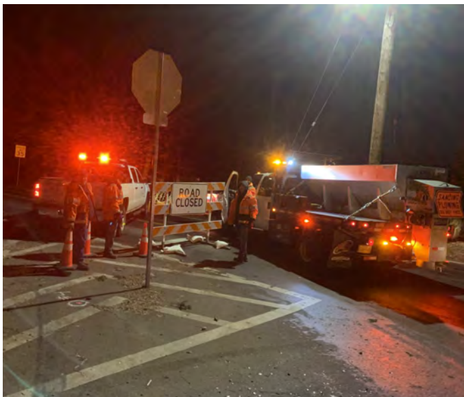
City of Gresham Transportation Operations crews set up a traffic closure to remove a tree that had fallen on the road. Dozens of trees blocked streets and downed utility lines during the storm.
